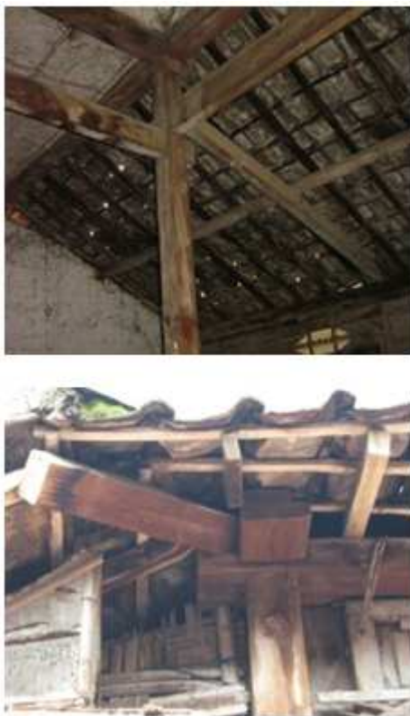
Picture 4.1. The house's original structure condition (Source: Susy Budi Astuti)
