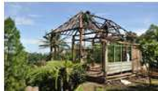
Picture 4.10. The Process of assembling soko and roof (Source: Susy Budi Astuti)
